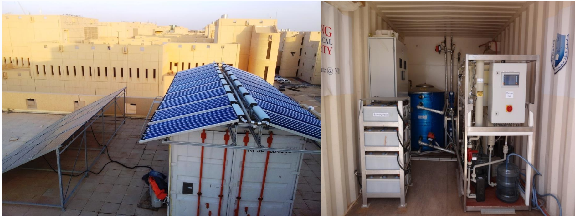
Figure 9. Picture of the portable solar-driven desalination system (at King Saud University)
